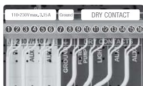
LIGHT Lighting control 1 & 2
